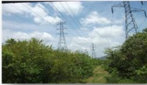
Fig 8: High voltage line within the MNP area
