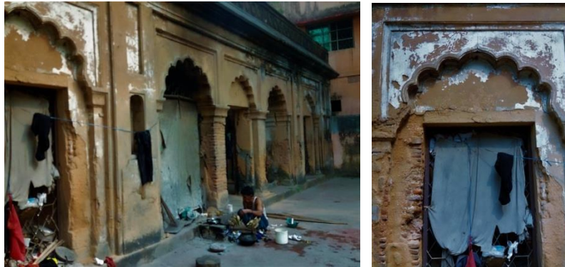
Figure Shows Present Condition of Bibi Mariam Guest House.
