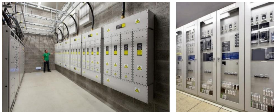
Fig. 9. HEMP filters (left) and control cabinets (right). For size comparison.
