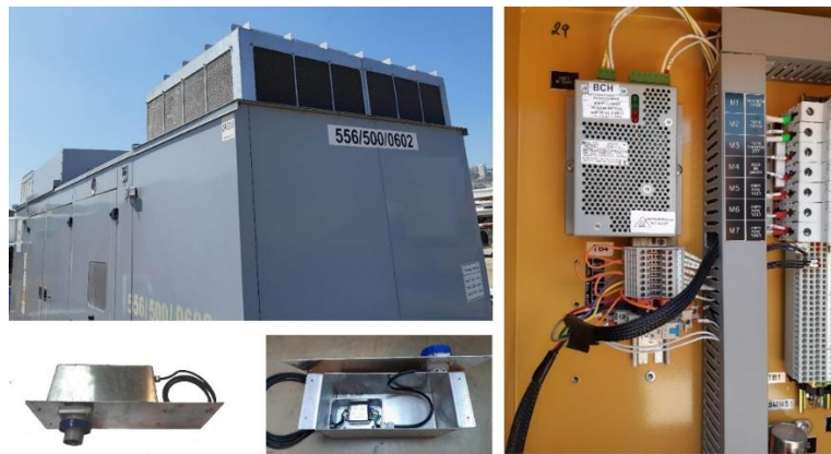
Fig. 30. Protection elements of the backup diesel generator, developed by the author.
