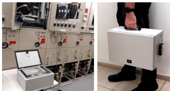
Fig. 25. HEMP protected backup power supply for electronic equipment testing after HEMP impact
