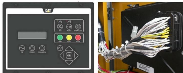
Fig. 29. Main controller of diesel generator
