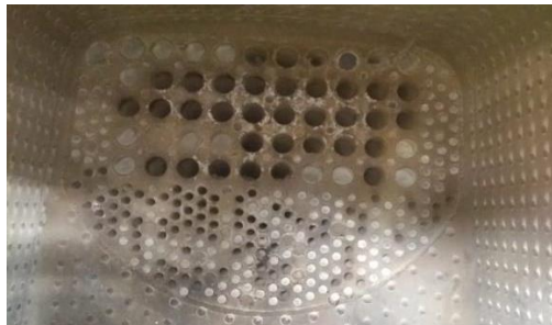
Figure 7: shows some blocked fire tubes of wood- fire tube boiler due to ash deposits
