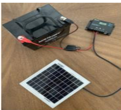
Fig6. 5W Solar Panel Charge a 12V Battery
