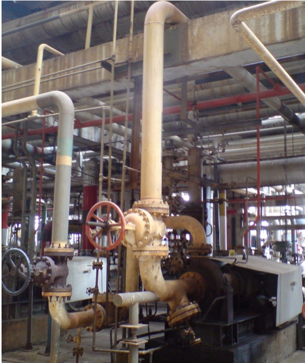
Fig. 2: Photograph of Naptha Stabilizer Overhead Refined LPG Product Pump Unit
