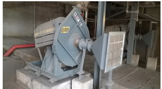
Fig. 13: Photograph of Scanner Fan Unit for Boiler
