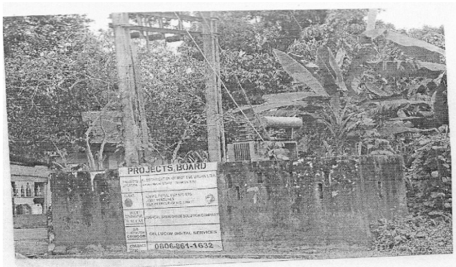
Plate IV: Electricity supply unit, a core Peri-urban facility providing electricity for the study area as captured in Ibiaku Ikot Ese, Uruan Local Government Area. (see section 3.1.2)
